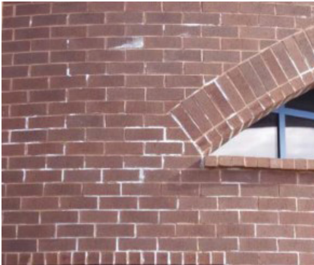
Photo 2 Efflorescence on Mortar Joints
