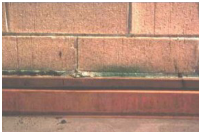
Photo 12 Stain from Copper
