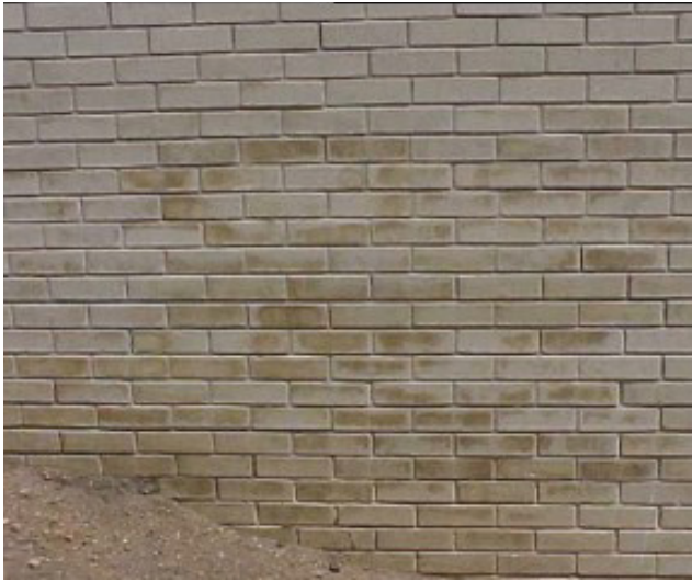
Photo 7 Yellow Vanadium Stain
