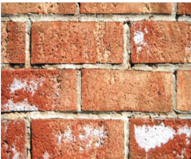
Photo 3 Efflorescence in Limited Areas
