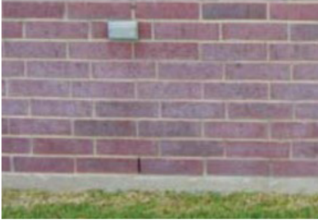
Photo 14 Hard Water Stain
